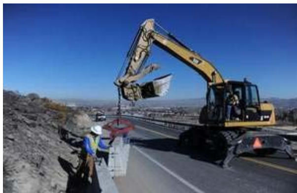
Workers install barriers along Lakeside Drive in the Bartley Ranch-Windy Hill area to guard against falling rock on the steep land burned by the
